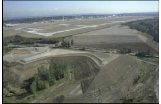
Third runway embankment construction at Seattle-Tacoma International Airport, 2002 Courtesy Port of Seattle
