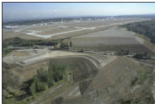
Third runway embankment construction at Seattle-Tacoma International Airport, 2002 Courtesy Port of Seattle
